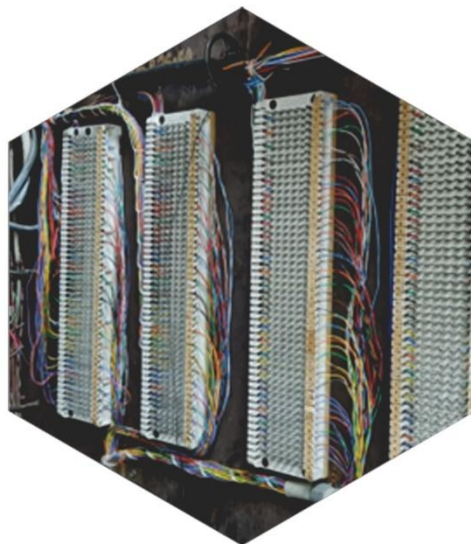
Phase 4 Upgrading of PABX Systems from Current Philips S1000 to New Philips SOPHO IS3070
